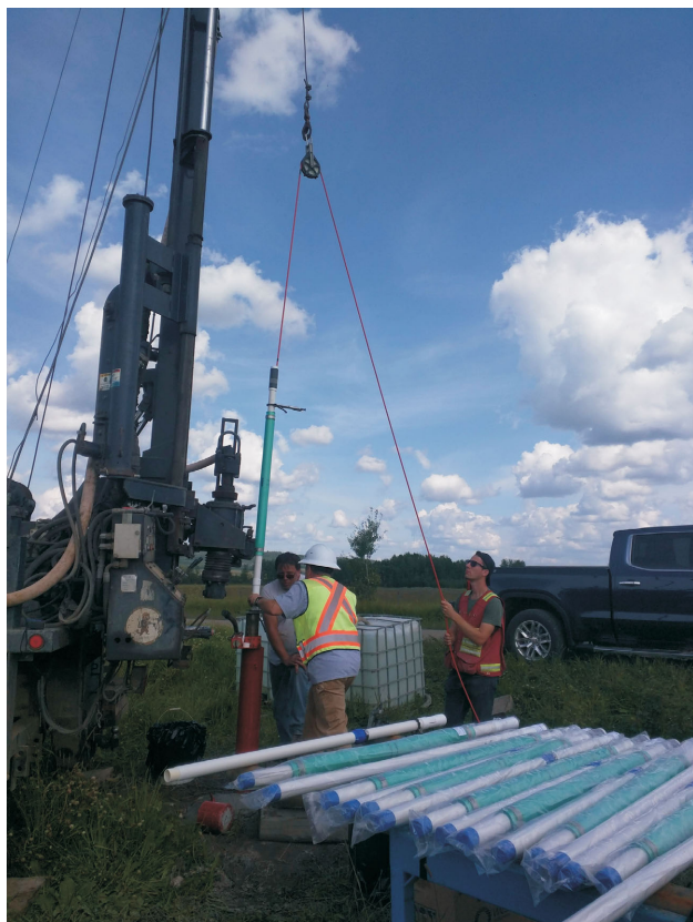
Figure 4. Installation of Westbay Instruments system in well EERI-11. The foreground shows the layout of the packers (green) and casing with measurement and pumping ports (white casing) during installation.
