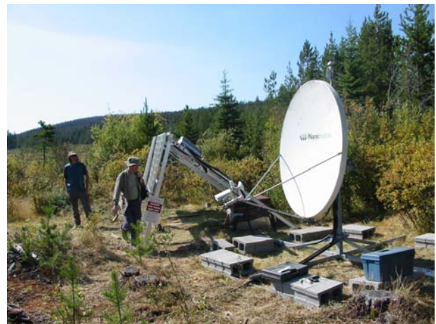
Figure 3. Photograph of Nechako seismic station RAMB, showing the typical station layout, with solar panels and a satellite dish (seismic vault is not visible).
